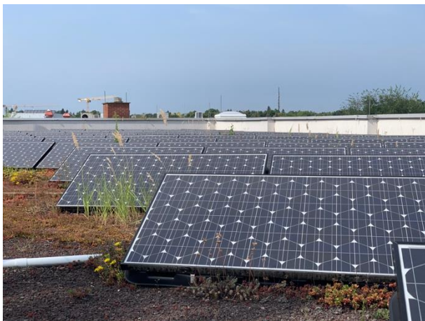
FIGURE6 Photovoltaic system on the roof
